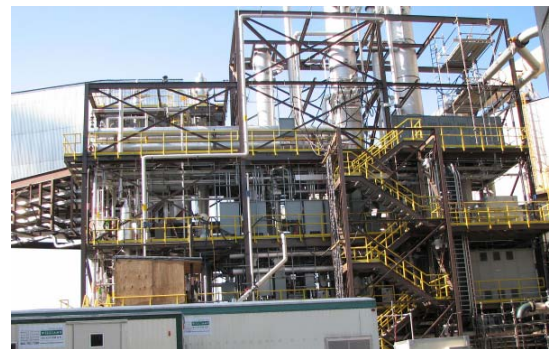
Figure 8 Field Pilot at We Energy's Pleasant Prairie Power Plant
