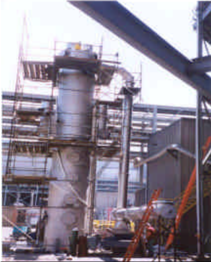
10,000 cfm wet ESP unit at Bruce Mansfield plant
