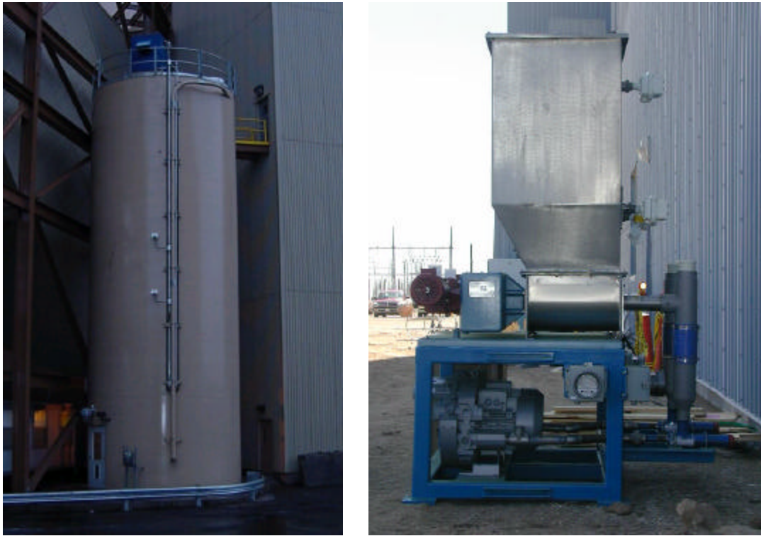
Figure 2. Carbon Injection Storage Silo and Feeder Trains for 150 MW Unit.
