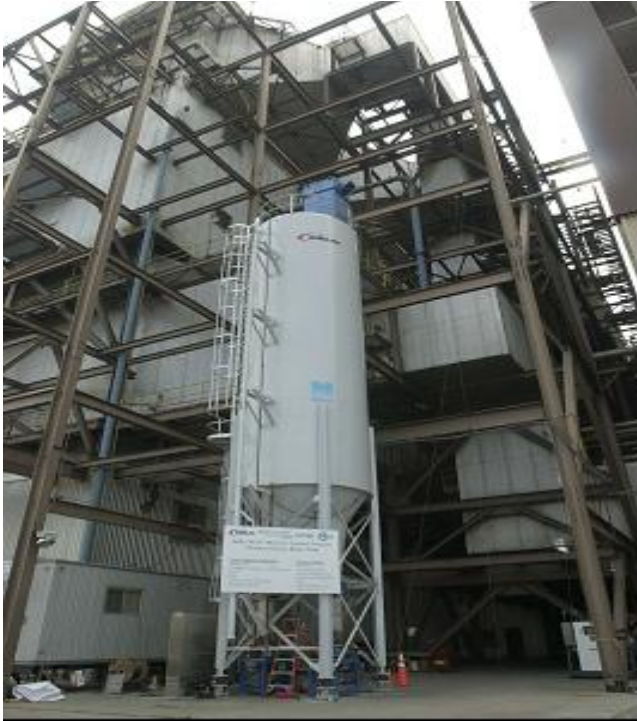
Figure 7. Carbon Injection Storage Silo and Feeder Trains for 150 MWs Fabric Selection
