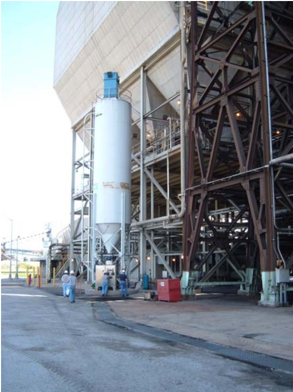
Figure 4. Long-Term Test Injection Silo.
