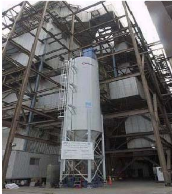
Figure 7. Carbon Injection Storage Silo and Feeder Trains for 150 MW.
