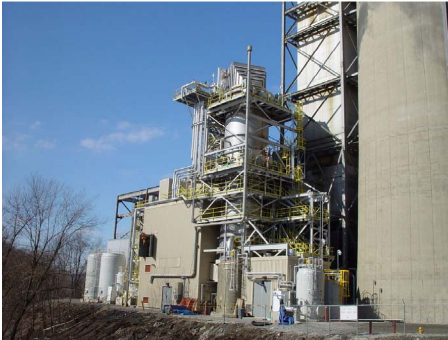
Figure 8. 50-MW ECO Commercial Demonstration Unit at FirstEnergy's R.E. Burger Plant
